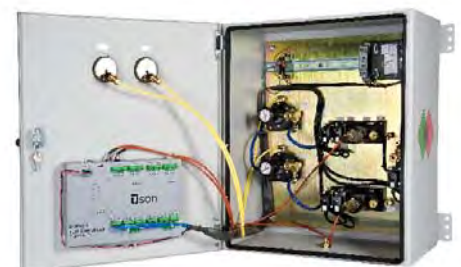
TCU2 is installed in pneumatics cabinet
